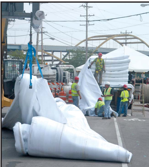
Workers prepare to line the inside of an older sewer to give it another 50 years of service life.
